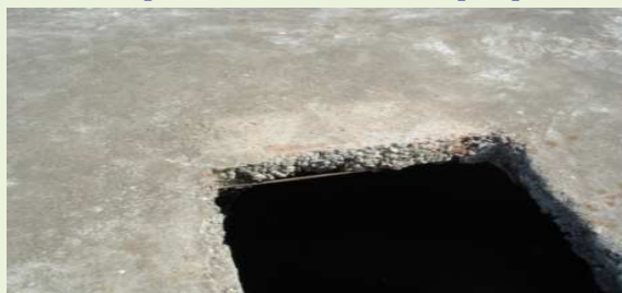
Sump without water vents
