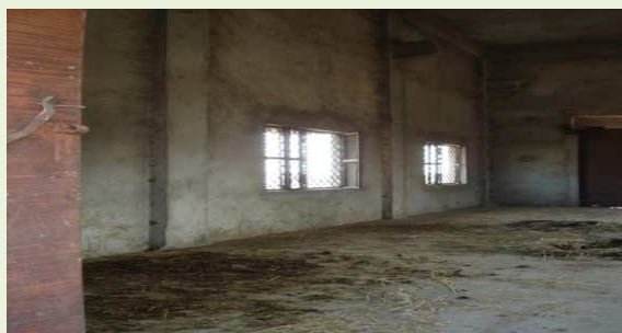
Pump house at Rudur without pumps
