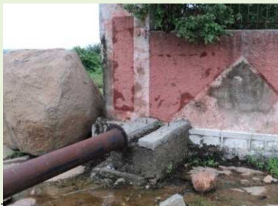
Pipeline from CPWS Vattinagulapally upto boundary wall of Osman Sagar Reservoir awaiting connectivity
