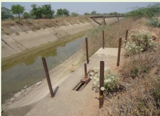
Sluice and Pump House at SRSP Canal (main source) lying Idle
